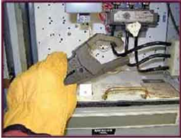
Figure 1. Installing a clamp-on current transducer.
